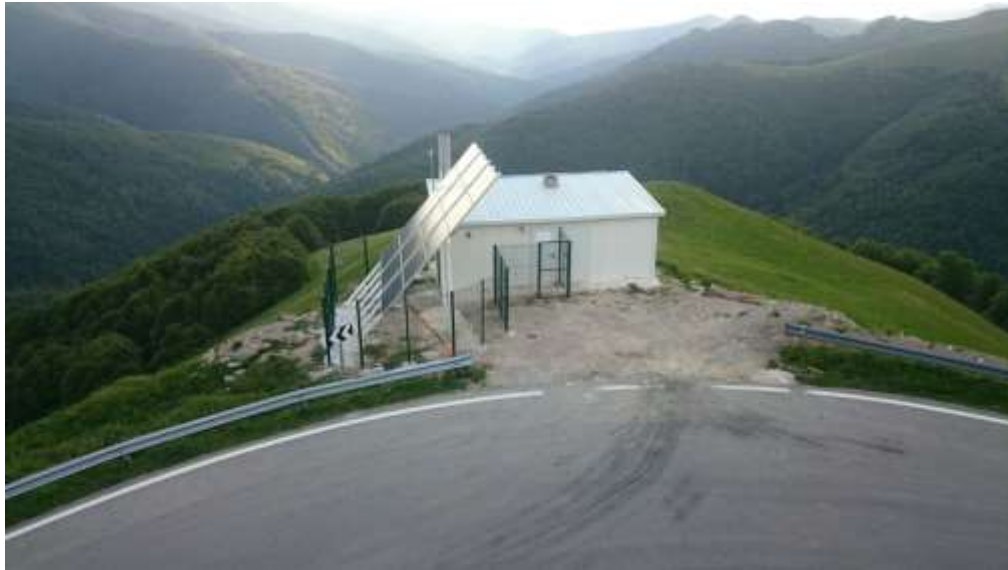
Figure 12: Abodi base station with solar panels located over Irati Forest
