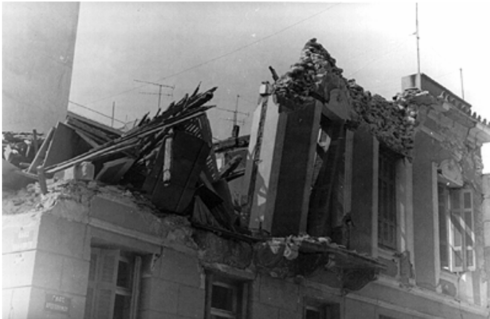
Photo 45: Hazardous, partially collapsed masonry building requiring urgent demolition
