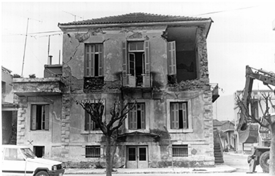
Photo 32: Partial collapse (RED)
