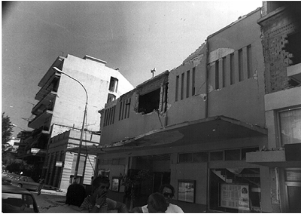
Photo 44: Partially collapsed wall and parapet, requiring urgent demolition
