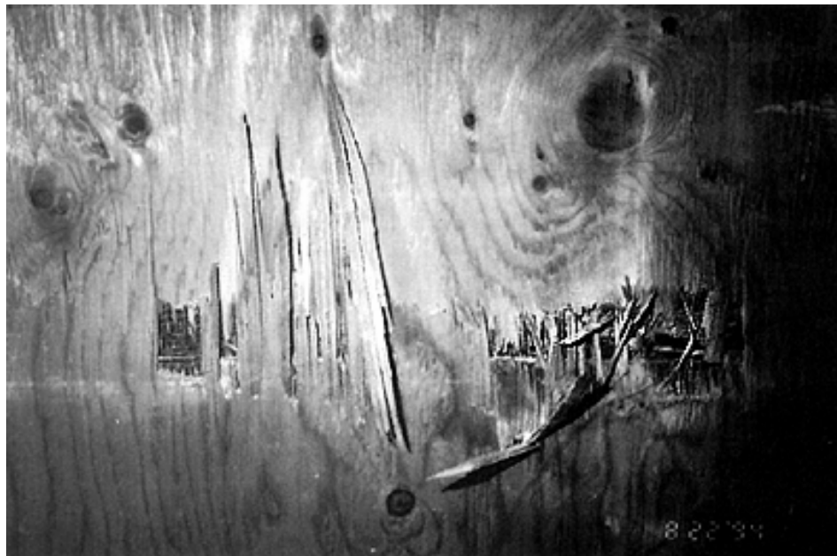
Photo 39: Local damage to plywood shear wall (YELLOW)
