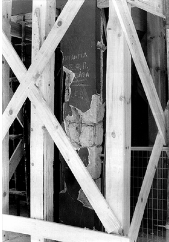
Photo 46: Emergency support due to failed column
