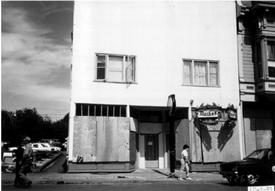
Photo 38: Damaged 2-storey wood frame building. Lots of broken glass and some lateral offset (YELLOW)
