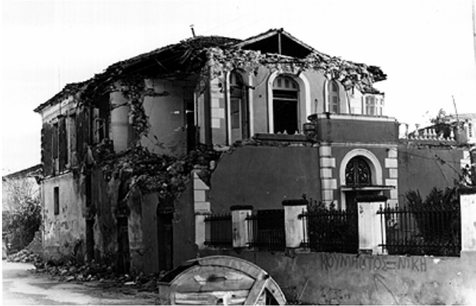
Photo 31: Partial collapse (RED)
