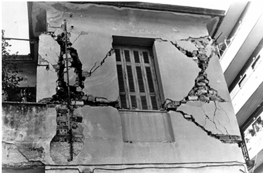
Photo 30: Severe damage (RED)
