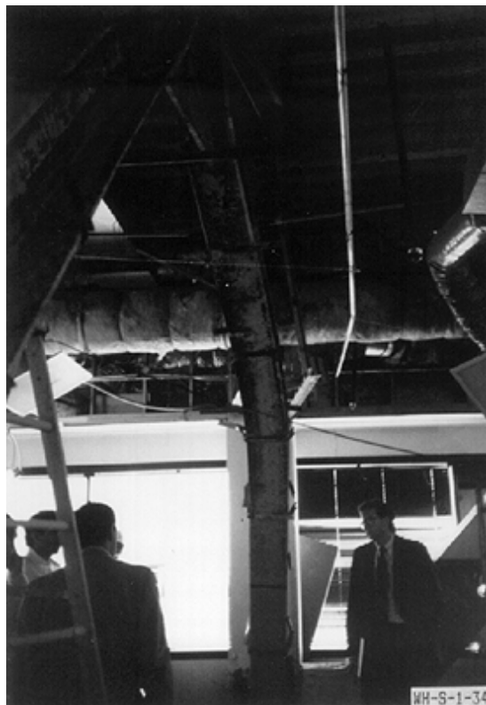
Photo 34: Buckled brace of building in Photo 29
