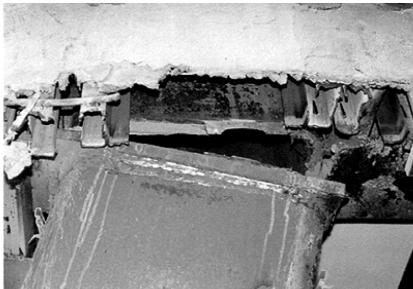
Photo 36: Fractured weld of the panel plate in beam-column joint (YELLOW)
