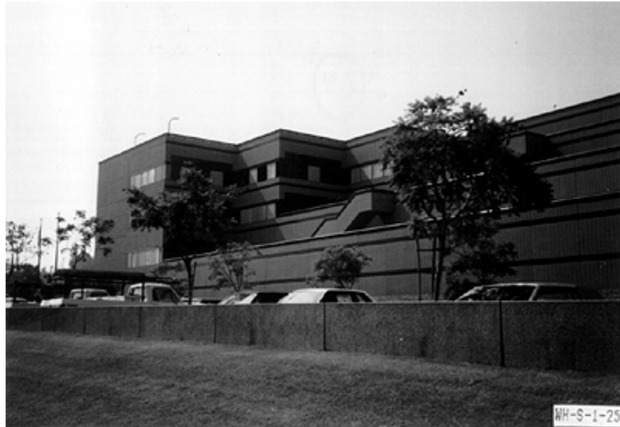
Photo 33: Four storey steel building with extensive broken glass and several buckled braces (YELLOW)
