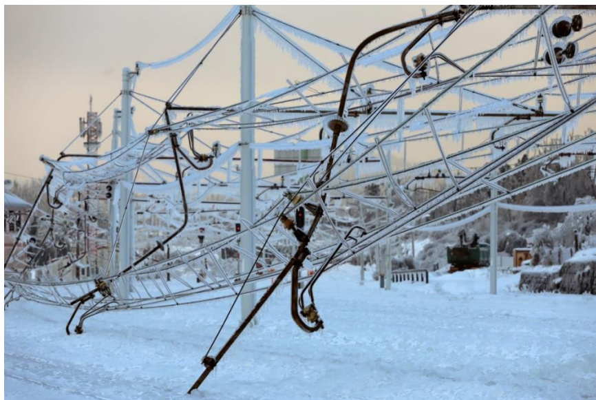
Figure 24: Sleet damage at Postojna train station
