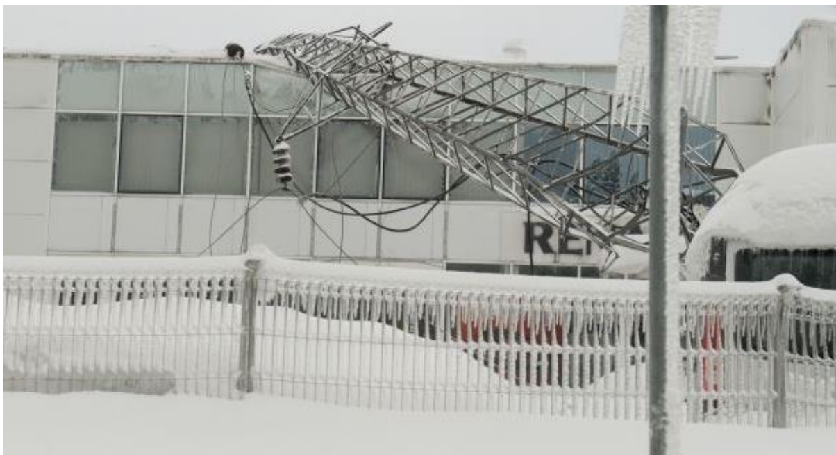
Figure 26: The consequences of fallen electricity lattice steel tower
