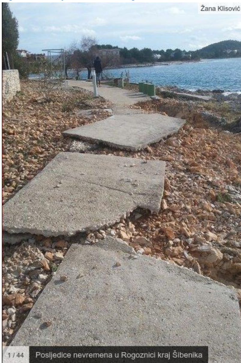
Figure 13: Destroyed waterfront in Rogoznica
