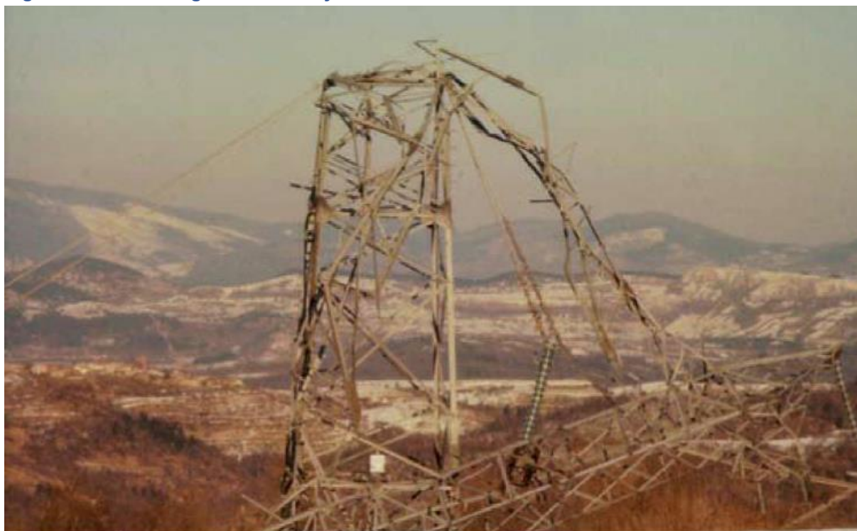
Figure 4: Sleet damage on electricity lattice steel tower in Brkini at the end of November 1980
