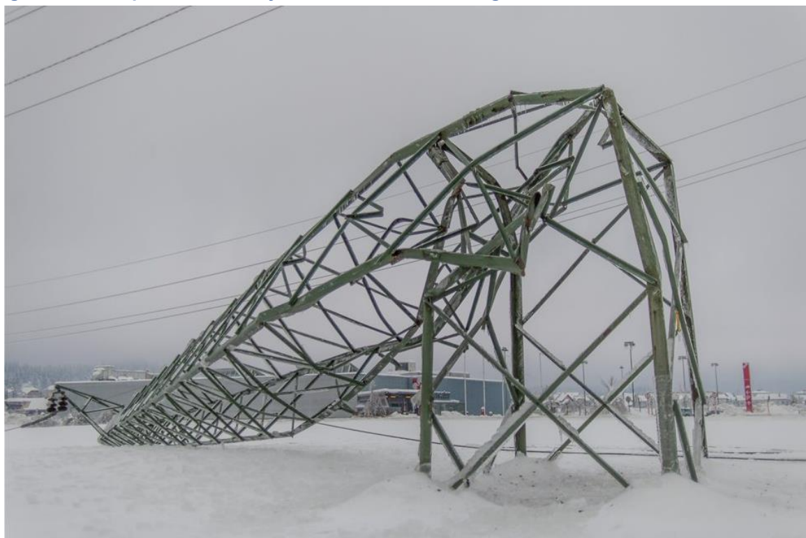
Figure 22: Collapse of electricity lattice steel tower in Logatec
