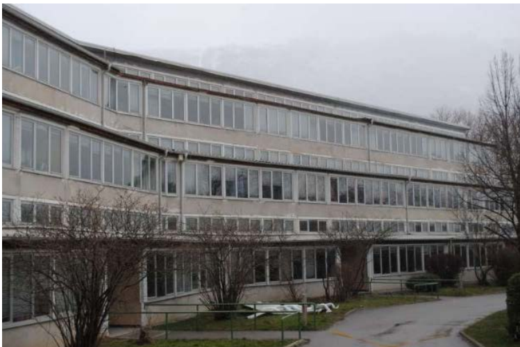
Figure 11: Wind damage school in Ajdovščina Municipality
