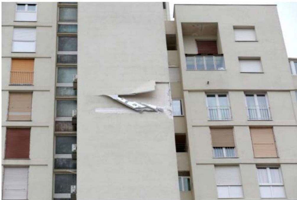
Figure 21: Damaged facade from strong Sirocco
