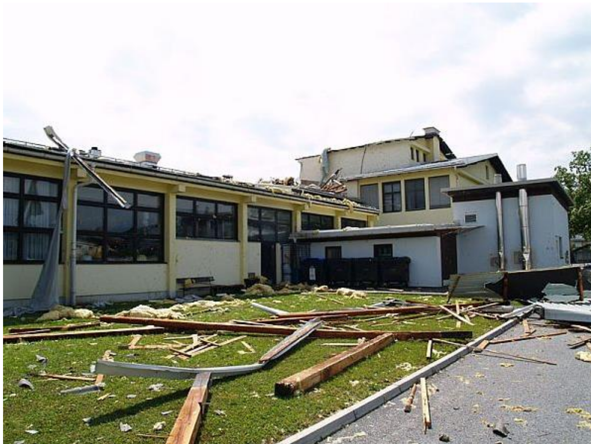
Figure 19: Damage on primary school Vodice.
