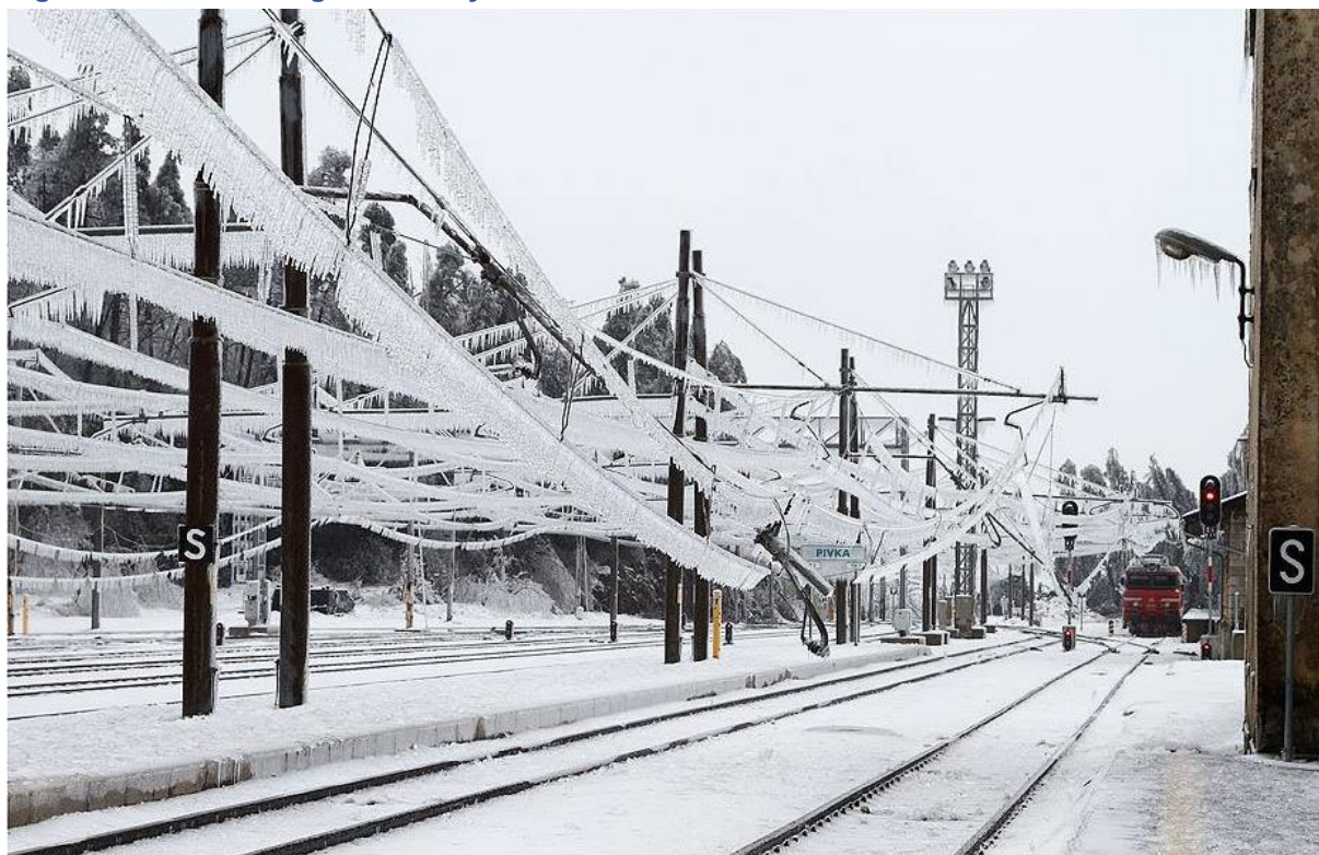
Figure 20: Sleet damage at railway station in Pivka
