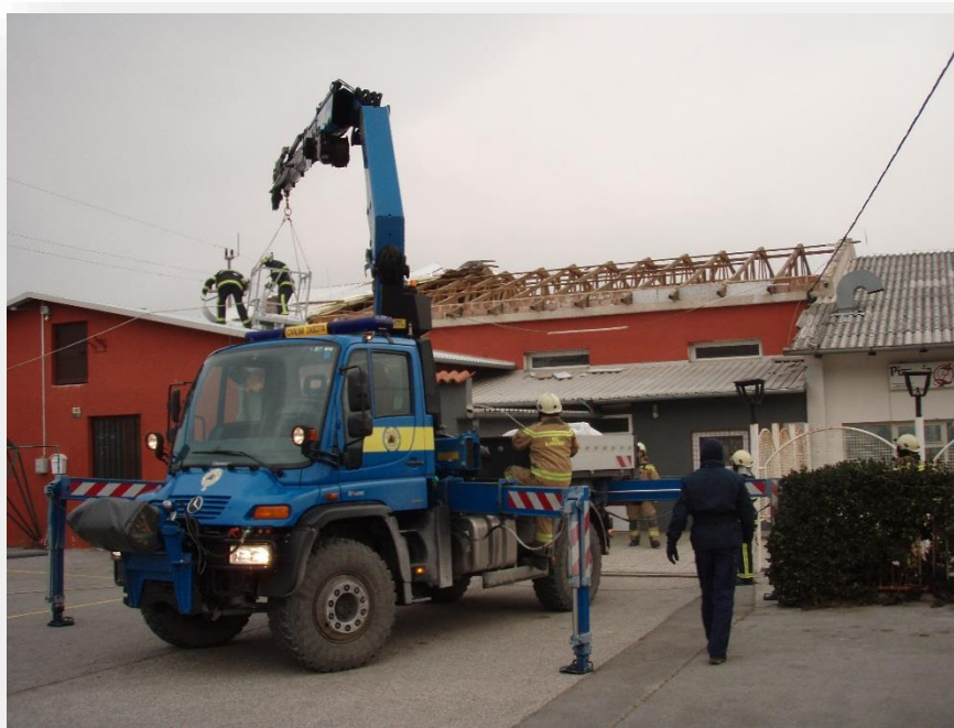
Figure 4: Wind roof damage
