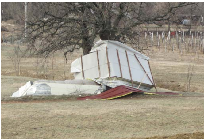
Figure 3: Torn off roof
