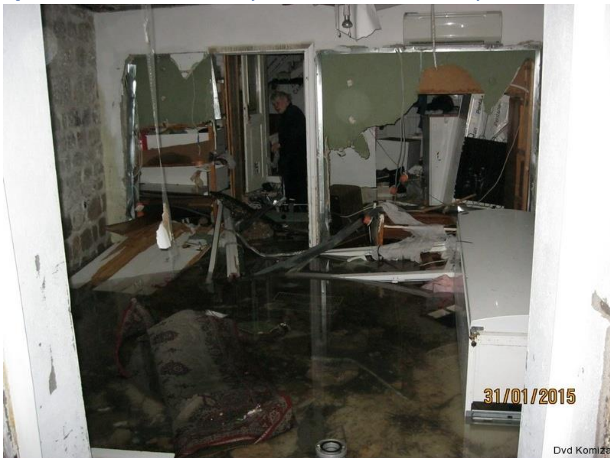
Figure 9: Debris from the waterfront destroyed the house wall, two women were injured inside the house
