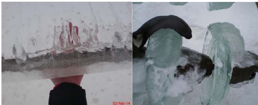
Figure 23: Amount of sleet on the conductor (left) and on the insulator (right)
