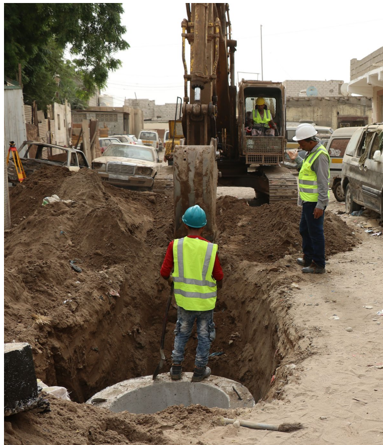
Workers are installing new sanitation pipes in Dar Saad district in Aden within the sanitation project implementation supported by UNICEF and the European Union. ©UNICEF Yemen 2019/ Mahmoud Fadhel
