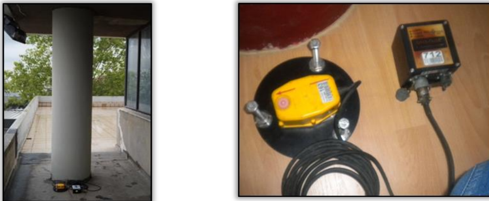
Figure 11 Installation of the temporary network in the buildings of the AUTH campus (see Figure 9). These sensors are located close to the RC columns.
