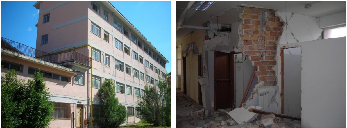
Figure 10 Façade (left) and damaged interior (right) of the investigated school building in L'Aquila, Italy.
