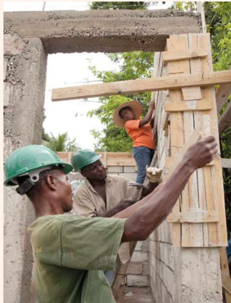
Trained builders and community members rehabilitating houses and public buildings in Haiti. © European Union - photo by EC/DG ECHO
