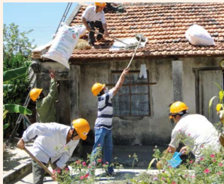
DWF-trained builders and families carry out household repairs in Vietnam. © European Union - photo by EC/DG ECHO/Evangelos Petratos
