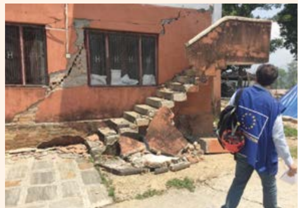
EU structural engineers assess hospitals and other key public infrastructure in Nepal. © European Union - photo by EC/DG ECHO/ Pierre Prakash
